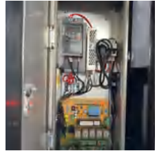
Electric control box
